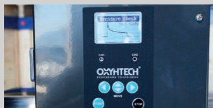
Checking the condition of the filter / differential pressure control
